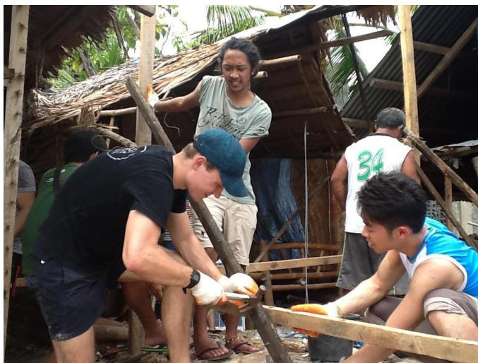
House construction in action [(From left to right) Jonas, Sam (a delegate from Silliman University in the
